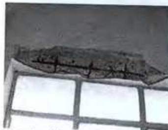
(iv) Spalling of Concrete from a Lintel (Location: Chittagong)
