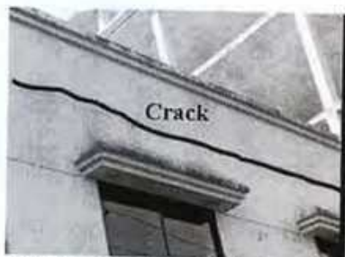
(iii) Cracks along the joint of parapet wall and roof slab (Location: Dhaka City)
