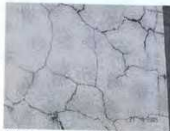
(ii) Cracks on the surface of a wall (Location : Dhaka City)
