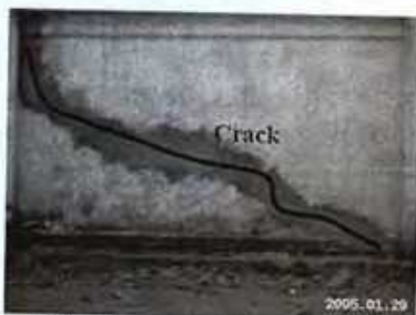
(i) Crack in a brick wall (Location: Dhaka City)
